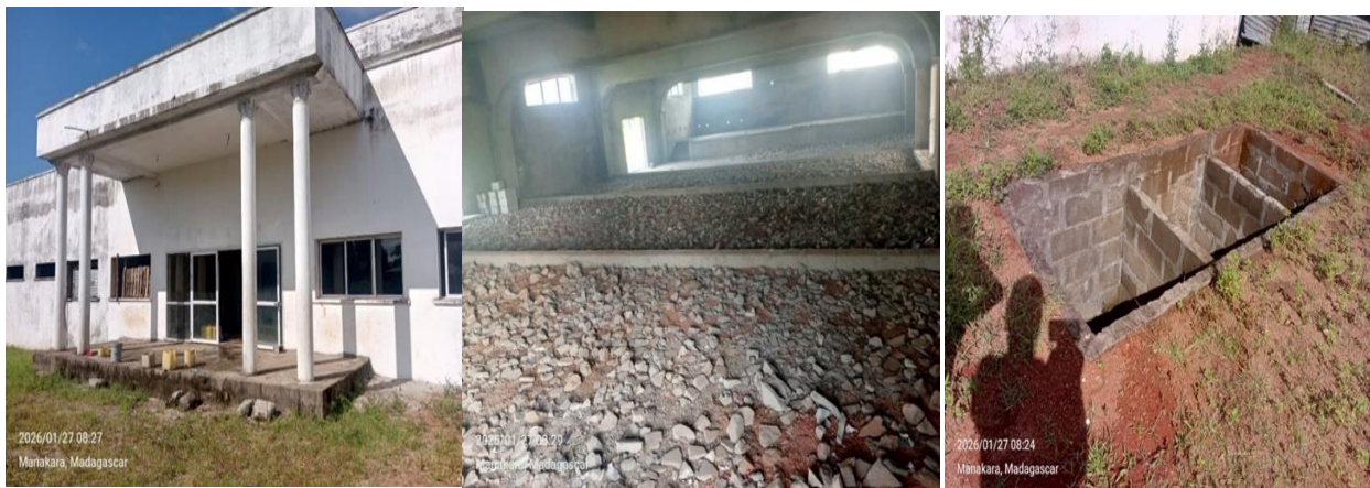
Figure 8: MCC de Manakara
