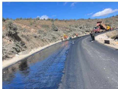
Figure 7: Insuffisance de signalisation et balise
